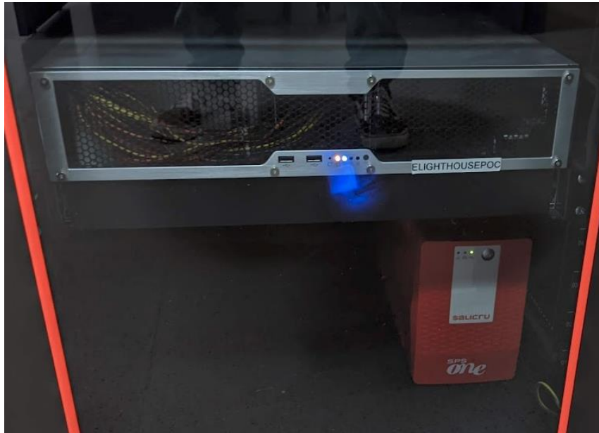
Figure 2.10 -- E-Lighthouse Server Rack
